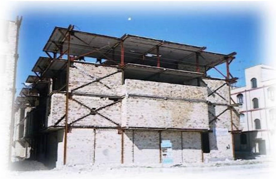
Figure 5 Soft story due to elimination of bracing in first story
