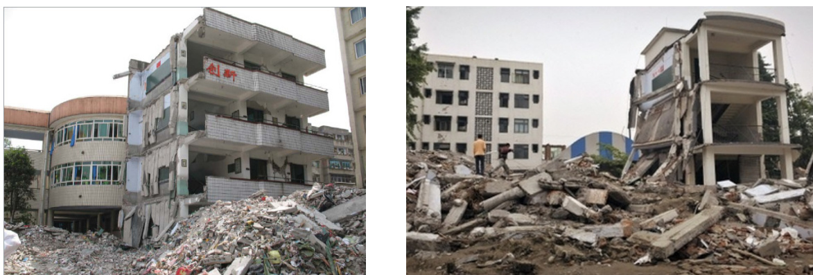
Figure 1 Collapsed school buildings from the 2008 Sichuan earthquake ( http://www.miyamotointernational.com/Sichuan/index.php )
