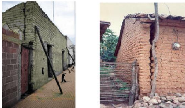
Fig. 5. Vertical breakdown in corners of adobe houses.
