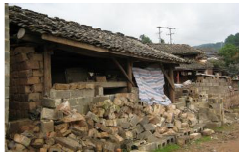
Figure 3. Partial collapse of residential house in Pu'er earthquake
