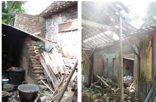
Figure 4. Most of buildings in Pundong made of brick and concrete, severed heavily damage.
