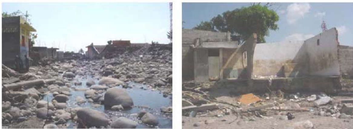
Figure 1. Damages in the constructions of Tapachula city, due to the Coatan river flooding during the Stan hurricane (Bitrán, 2006).
