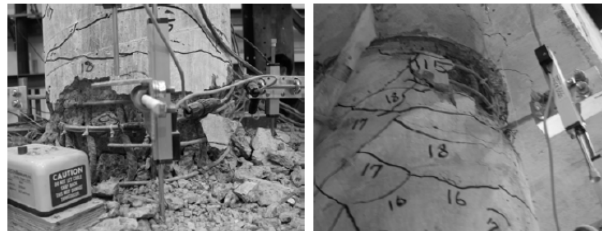
Figure 3 Damage Observed on the Lower and Upper Portion of Bent-3 after T-19
