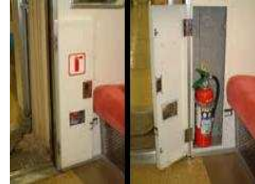
Fig. 6 Fire extinguishers in Busan subway train
