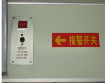
Fig. 4 Emergency button in Beijing subway train
