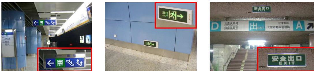
Fig. 9 Exit signs in Nanjing and Beijing subway station.
