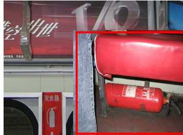
Fig. 5 Fire extinguishers in Beijing subway train
