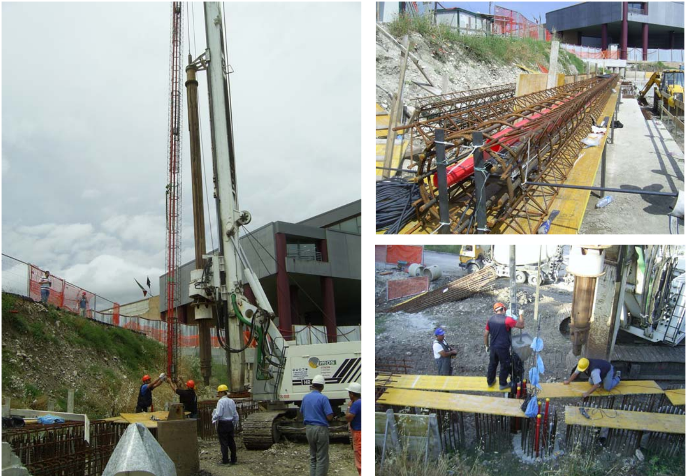
Figure 2 Installation of sensors (left) and the instrumented piles during preparation and concrete casting (right)
