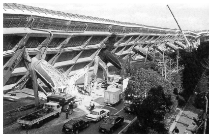
Fig. 4: Kobe, Japan, M=7.2, 1995: Collapse of Hanshin Line
