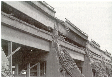
Fig. 1: Loma Prieta, U.S.A., 1989: M=7.1, Cypress Bridge Failure
