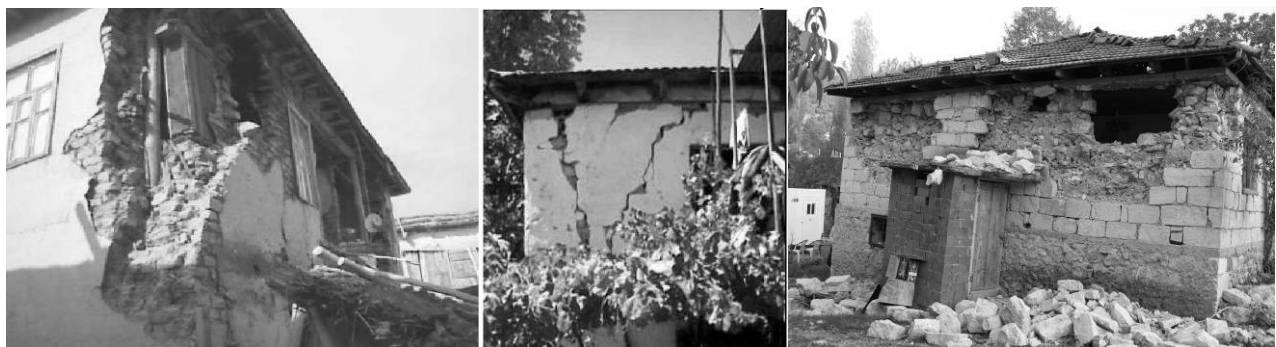
Figure 1. Damages observed in past earthquakes.
