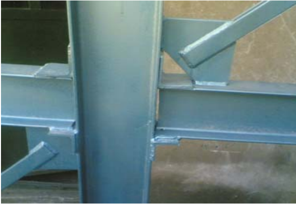
Figure 5. Connection plate with cut off corner to let the connections act as hinge connections
