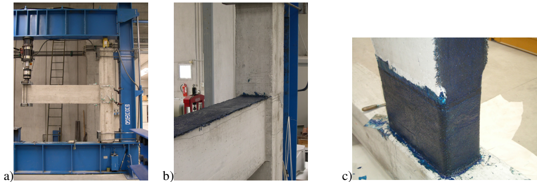
Figure 4 Experimental program at UNIUD RU, joints at real scale: a) test set-up with a joint, b) application of carbon fiber fabric at beam extrados, c) wrapping on beam close to column.
