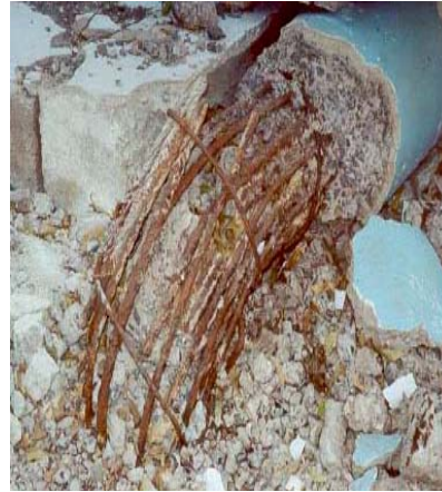
Figure 2 Collapsed column with inadequate lap splice length and widely spaced transverse bars (Gujarat, India, 2001)
