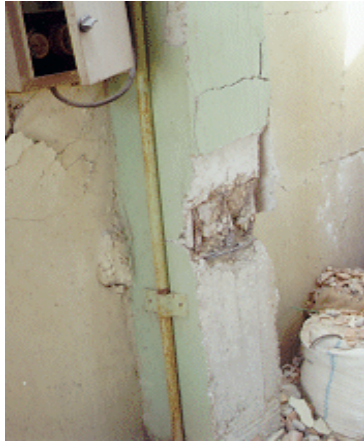
Figure 1 Damage in lap splice point caused by absence of adequate confinement and improper lap splice (Bingol, Turkey, 2003)
