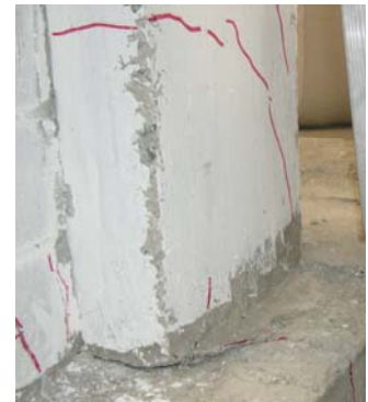
e) Evidence of rotation at the base of the compression column at 71.6mm
