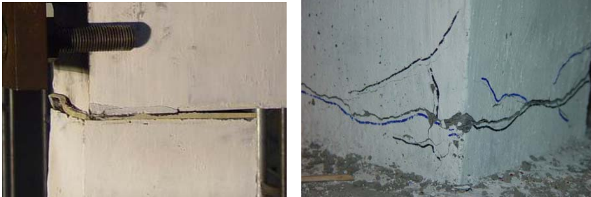
Figure 5 Extruded rubber cushion and breakages of column bottom
