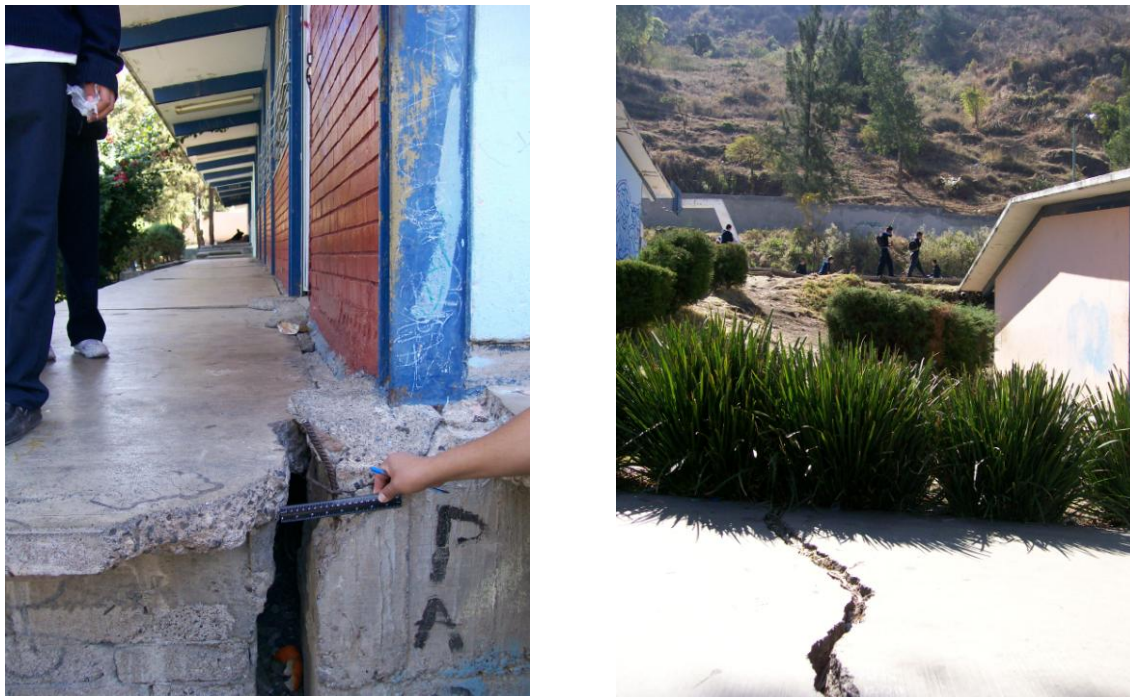
Figure 5 Middle School playground damages
