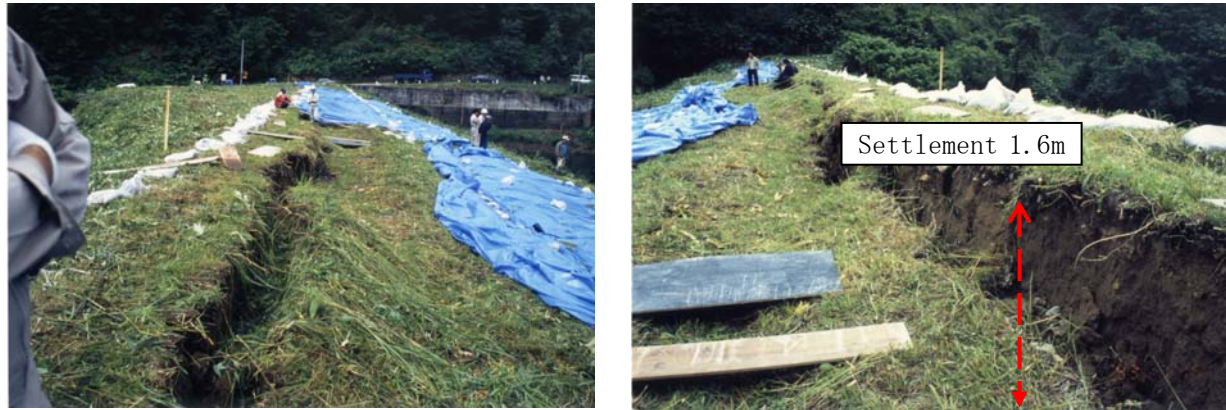
Figure 4 Damaged Niwa- Ikumine Dam (1993 Hokkaido-Nansei-Oki Earthquake)
