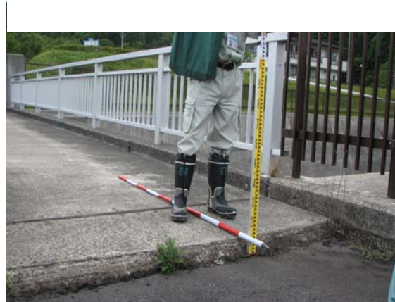
Figure 3 Faulting of approximately 10 cm at the interface between the natural ground and the dembankment on the right bank (2008 Iwate-Miyagi Inland Earthquake)
