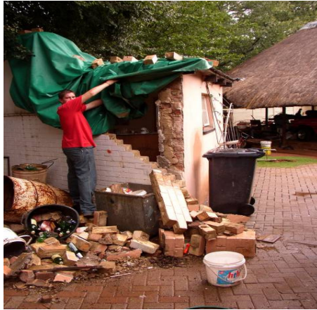
Figure 7: Failure at wall intersections without ties.
