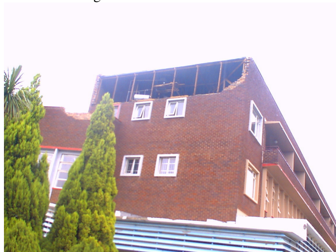
Figure 5: Out-of-plane failure of a gable.
