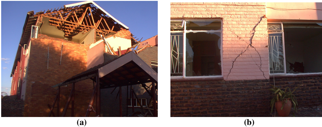
Figure 3: (a) In-plane and (b) out of Plane Response of the Bal Eaton Court building.
