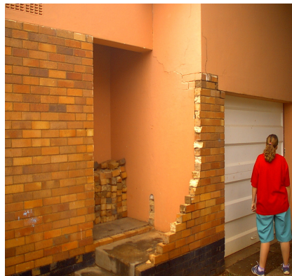
Figure 4: Failure of a cantilevered wall
