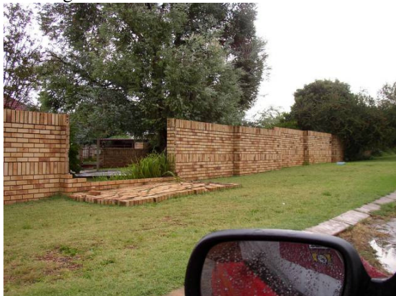
Figure 8: Collapse of an irregularly shaped wall section
