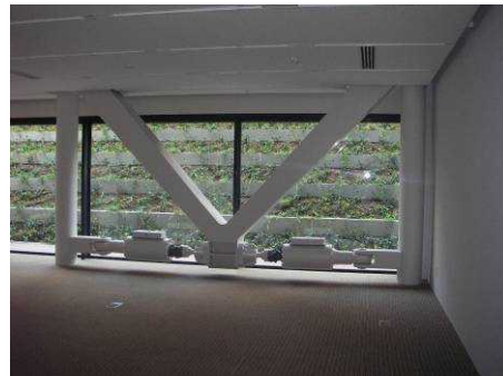
Figure 6: Oil dampers intensively provided on vibration control story
