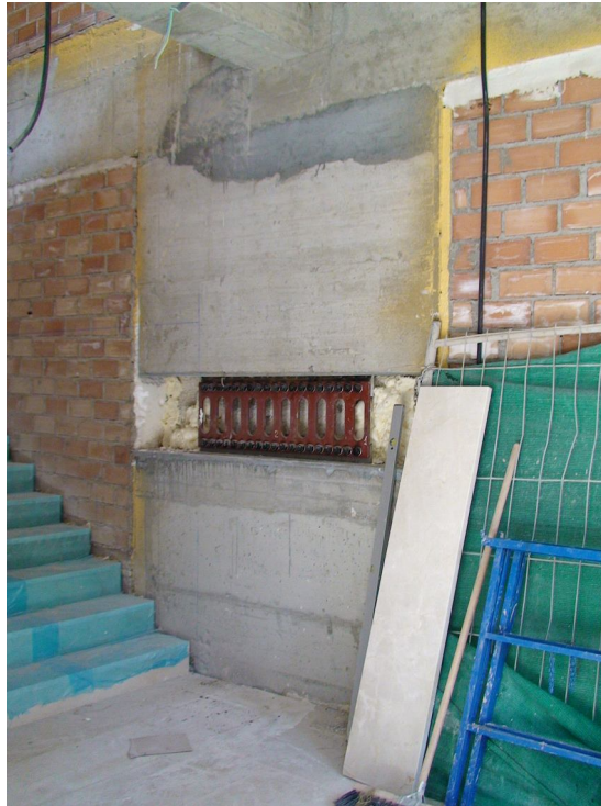
Fig. 5: Photograph of the energy dissipating devices in the first storey.
