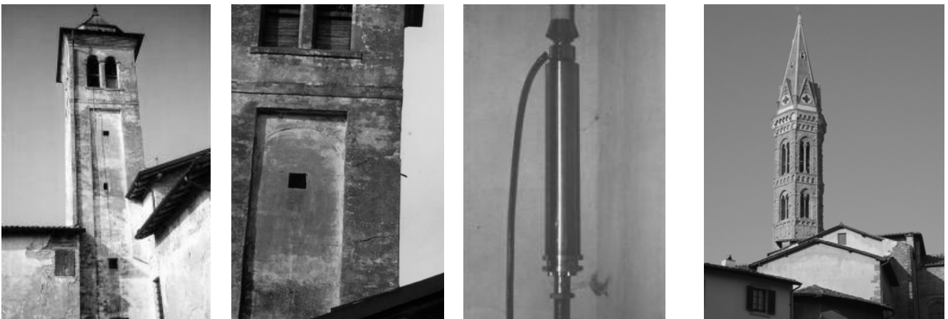
Figure 11 From left to right: (a-b) the Bell Tower of the San Giorgio in Trignano Church , cut into 2 pieces by the 1996 Reggio Emilia and Modena earthquake; (c) one of the 4 SMADs used in series to the vertical ties to retrofit the bell tower in 1999; (d) the Bell Tower of Badia Fiorentina at Florence, seismically improved with 18 SMADs in series to ties in 2006.
