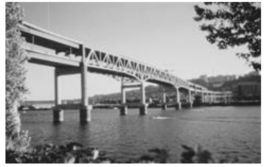
Figure 20 Marquam Bridge , Oregon (USA), retrofitted with Italian isolators and EPDs (centre, below).
