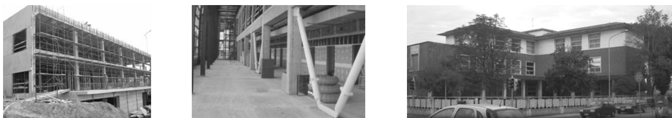
Figure 9 (a-b) Left and centre: views, during construction in 2005, of the new building of the Polytechnical University of Marche at Ancona (seismic zone 2), protected by 86 Buckling Restrained Braces (BRBs). (c) Right: Perticari High School at Senigallia (Ancona, seismic zone 2), rationalist architecture like the Gentile Fermi School of Figure 8, recently seismically retrofitted with dissipative braces, because of its bad concrete quality and non-symmetric shape.
