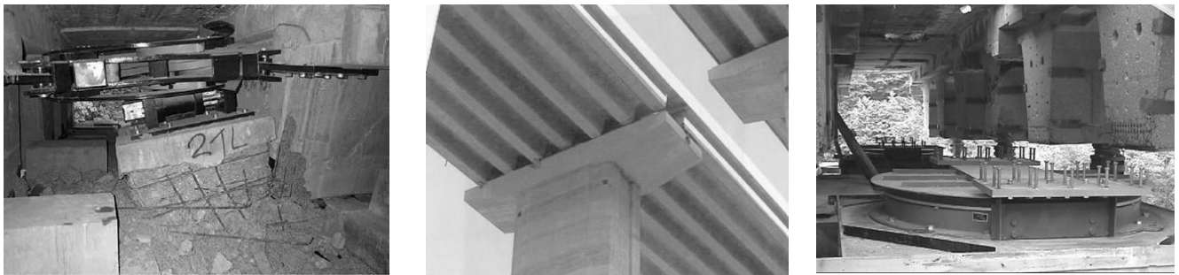
Figure 2 An EPD of the viaduct of Figure 1 (left) and its deck hardly still supported by some very inclined piles (centre) just after the 1999 Duzce earthquake. Right: one of the Friction Pendulum System (FPS) devices that were later used to retrofit the viaduct (usually 700 mm diameter, but 900 mm diameter at fault crossing).
