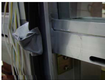
(a) Slippage of glazing bead
