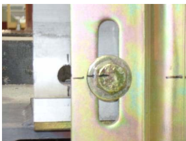
(a) Fastener slippage
