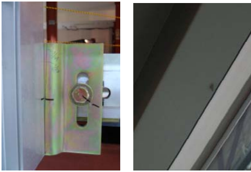
(a) Rotation of a fastener bracket (b) Disengagement of a screw at the blind box Photo 3 Damage of Case 3)
