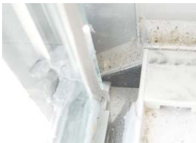
(a) Some defects at glass corner
