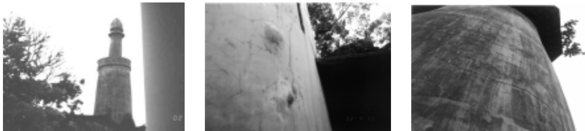
(a) inclined pagoda (b) protruding of partial wall and vertical cracks (c) lateral cracks
