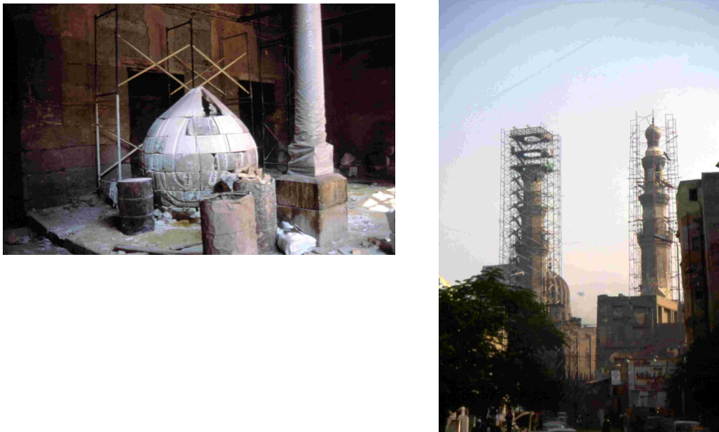
Figure 3 Pictures of minarets of Prince Shaykhou during restoration after the October 12, 1992 earthquake.
