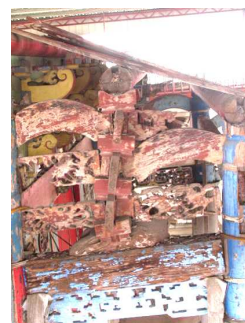
Figure 3 Failure mode of Dou-Gon joint set
