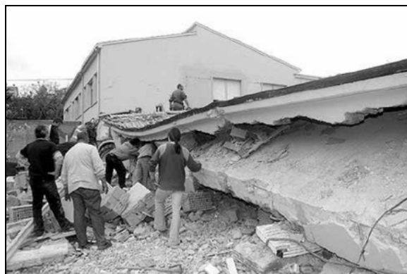
Figure 1 School collapsed in S. Giuliano village - earthquake M=5,4
