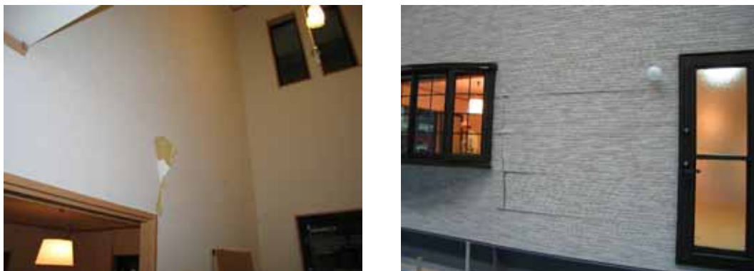
Photo 3 Damage of check third (Left: Inside, Right: Outside)
