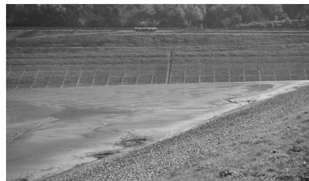
Figure 5 Boiled Sand indicating Liquefaction
