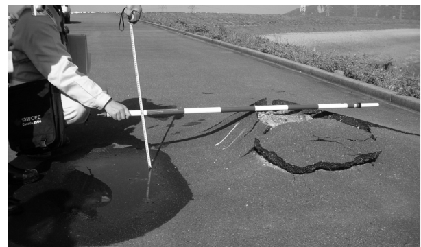
Figure 4 H-beam's Top indicating Settlement
