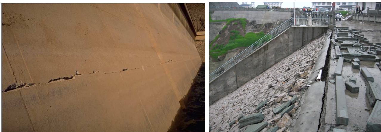
Fig. 2: Damage in top portion of the 105 m high Sefid Rud buttress dam caused by the magnitude 7.5 Manjil earthquake in Iran in 1990 (left), damage in concrete face of Zipingpu concrete face rockfill dam caused by the magnitude 8 Wenchuan earthquake in China in 2008
