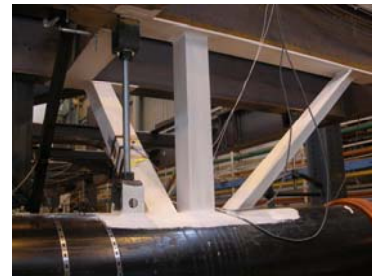
Figure 2(c) Rigid seismic bracing
