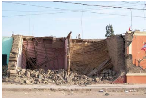
Figure 2 Adobe walls along the street frontage have collapsed. (D. C. Hopkins)
