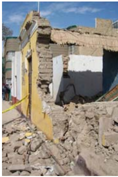
Figure 1 Partially collapsed adobe house. (D. C. Hopkins)
