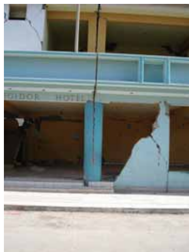
Figure 11 Detail of column failure
