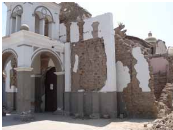
Figure 4 Damage in an adobe church
