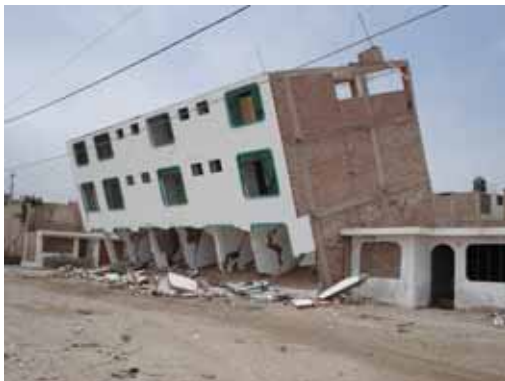
Figure 8 Failure of north side columns
