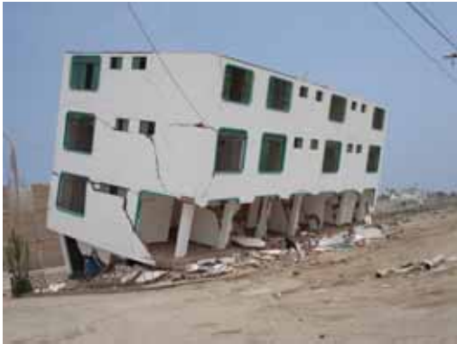
Figure 6 Collapse of 1 st floor of a masonry building
