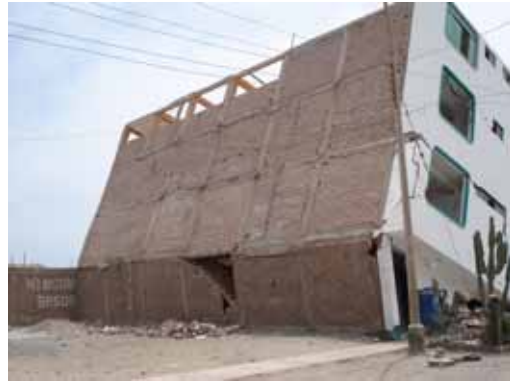
Figure 7 South view of collapsed building
