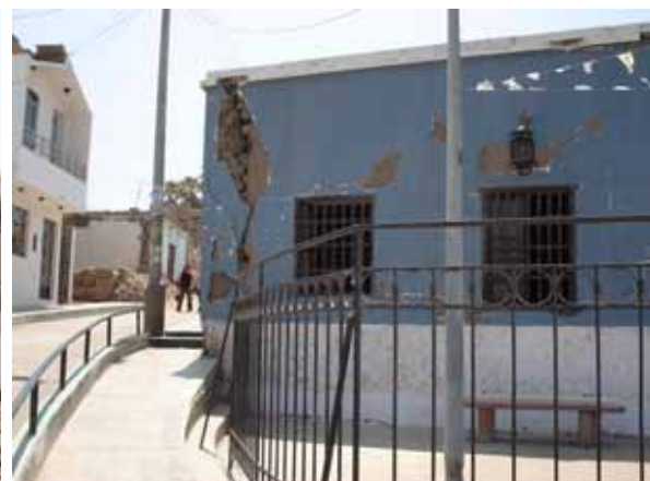
Figure 5 Typical failure of adobe construction
