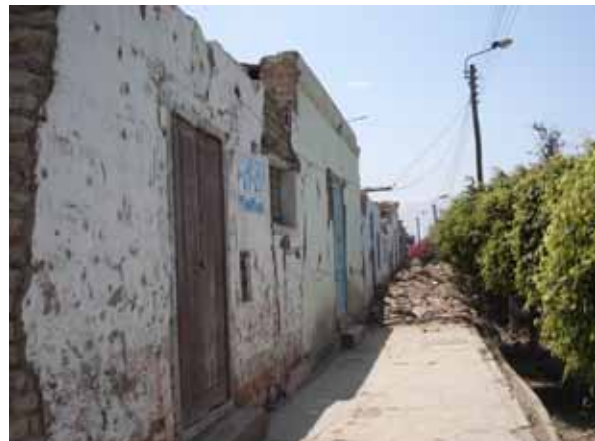
Figure 3 Damage in a group of adobe houses
