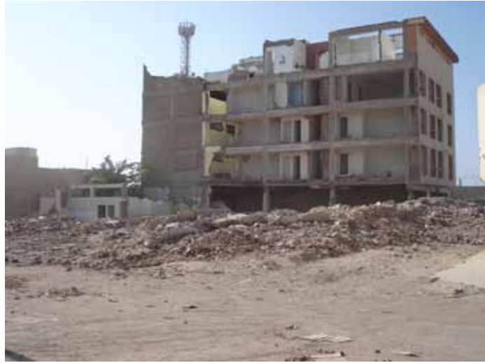
Figure 13 Collapse of five stories hotel
