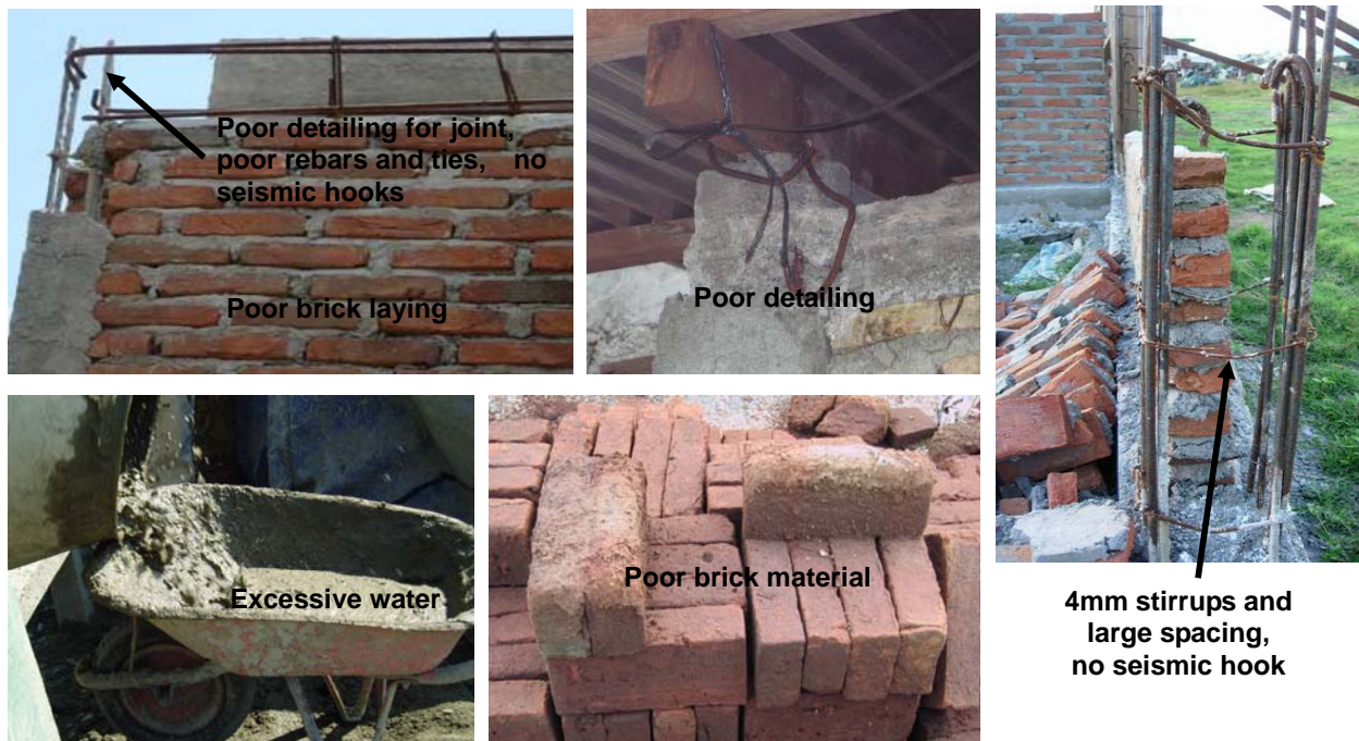
Figure 1 Problems in quality of material and construction techniques
