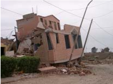
Photo 11: Collapse due to soft story
