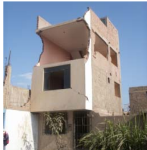
Photo 6: Damage on wall
