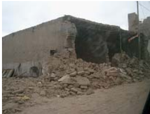
Photo 1: Overturning of walls
