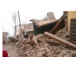
Photo 3: Collapse of roof
