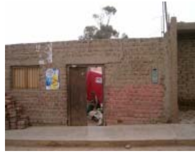
Photo 15: Internal collapse of adobe house
