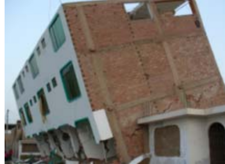
Photo 10: Collapse due to irregularity
