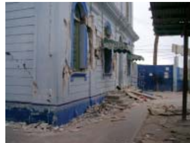
Photo 11: Failure because non reinforce
