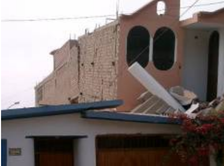
Photo 9: Collapse due to cut on belt beam
