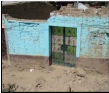
Photo 18: Collapse in Huaytara
