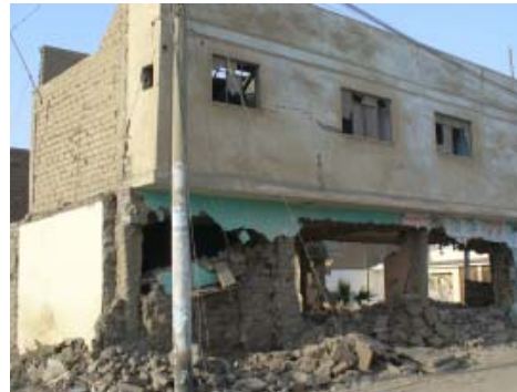
Photo 13: Mix structure – Failure on adobe
