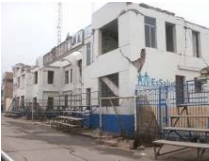
Photo 12: Damage ESSALUD Hospital
