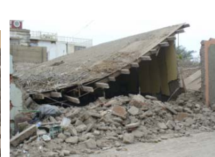
Photo 4: Collapse of wood roof
