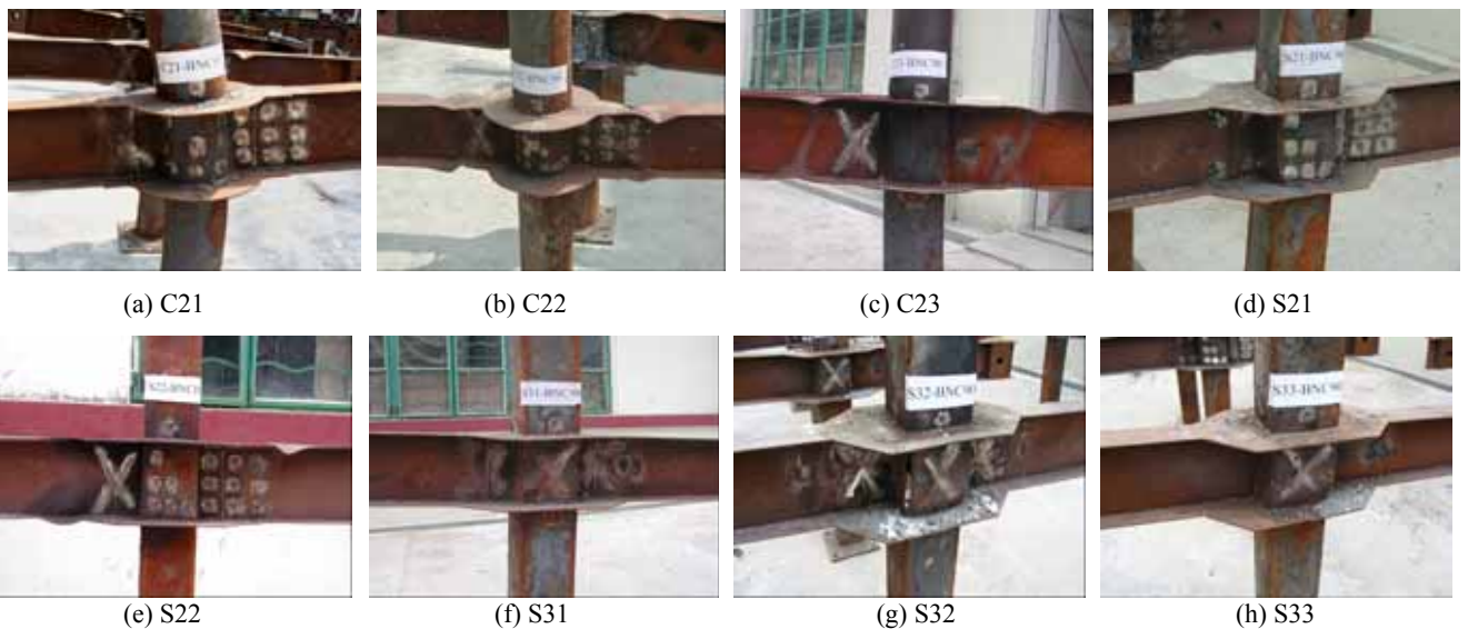
Figure 3 Joint specimen failure mode
