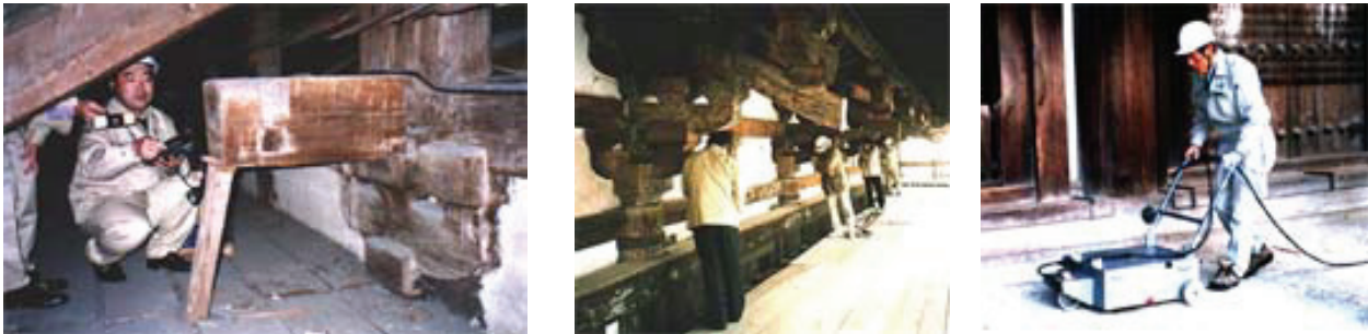
Figure 6.2 Example of deterioration and structural investigation
