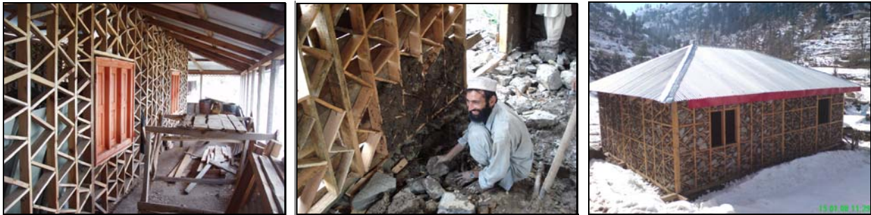
Fig.5: House in Bagh-Topi, Kashmir; Fig.6: Stone and mud infill; Fig. 7: Demo house after training in Jared, Kagan valley
