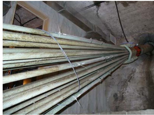
Figure 9: SOFO sensors, cable section in the anchorage chamber.
