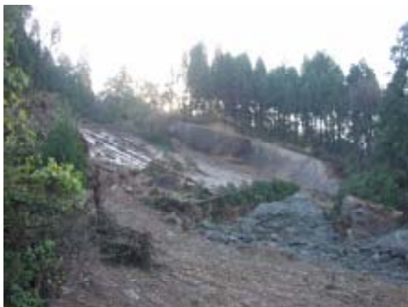
(a) Whole of collapse
