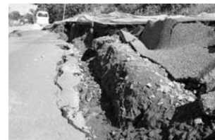
(b) Tonowa : Crack and scarp due to landslide of steep slope
