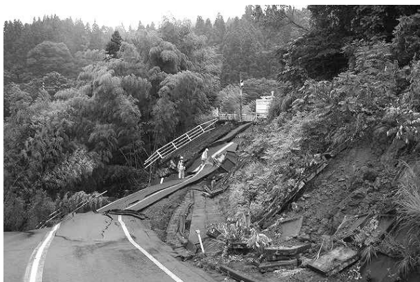
Photo 1 Ozumi, Nagaoka: Landslide at Route No.8
