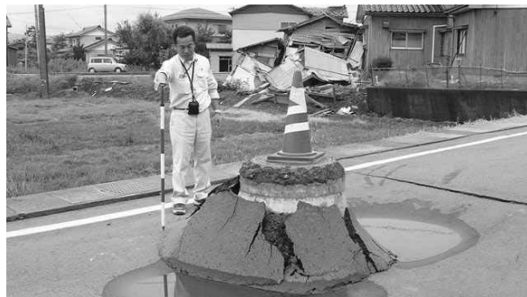
Photo 18 Uplifted sewer manhole (Photo: By Hiroyoshi Kiku)
