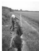
(d) Machikarui, Teradomari: Crack at high water channel of the Shinano River (Photo: BY Shinanogawa River Office, MLITT)
