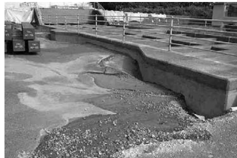
Photo 16 Settlement and apouted sand at Kashiwazaki Kariwa Nuclear Power Plant
