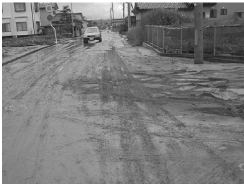
Photo 8 Street covered by spouted sand
