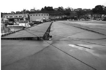
Photo 5 Inclination of caisson quay and trace of sand pumping at Kashiwazaki Port
