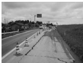
(c) Machikarui, Teradomari: Crack in left bank of the Shinano River (Photo: By Shinanogawa River Office, MLITT)
