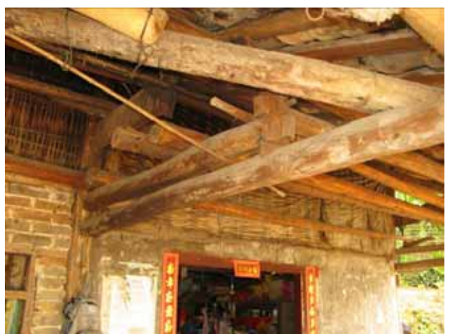
Figure 10 Brick-wood structure, Ms 8.0 Wenchuan Earthquake
