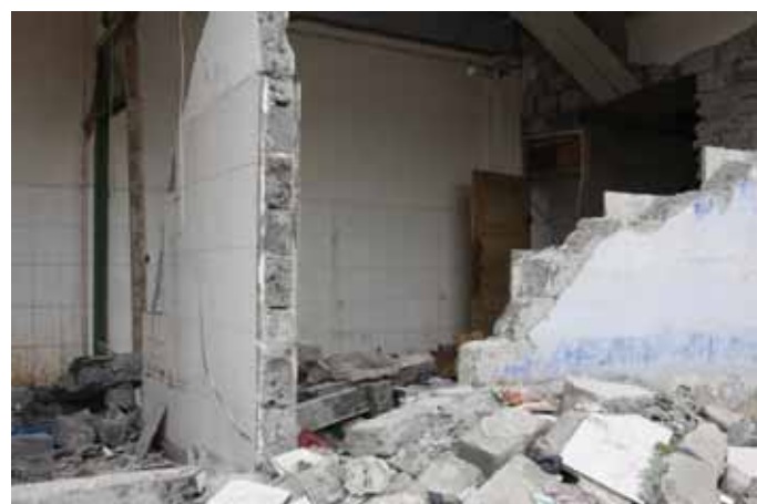
Figure 4 Brick structure, Ms 8.0 Wenchuan Earthquake
