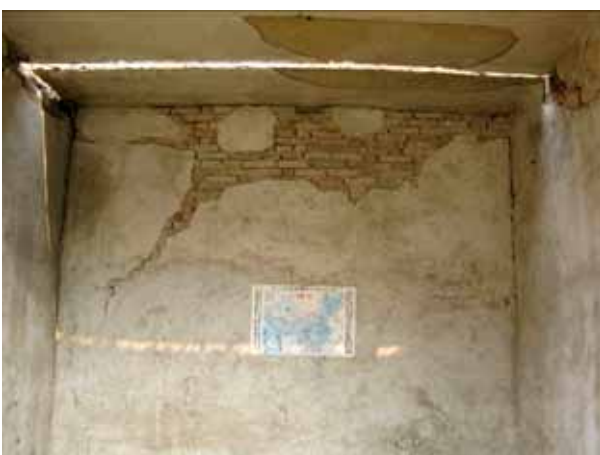
Figure 3 Brick structure, Ms 8.0 Wenchuan Earthquake
