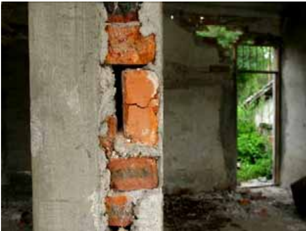
Figure 5 Brick structure, Ms 8.0 Wenchuan Earthquake
