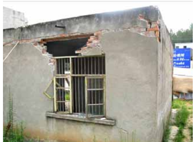
Figure 2 Brick structure, Ms 8.0 Wenchuan Earthquake
