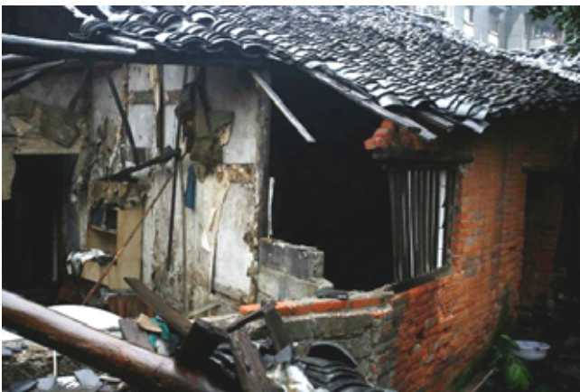
Figure 7 Brick-wood structure, Ms 8.0 Wenchuan Earthquake
