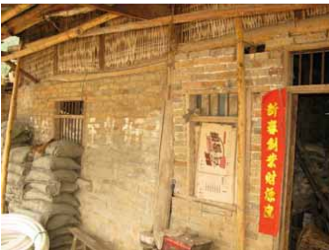
Figure 9 Brick-wood structure, Ms 8.0 Wenchuan Earthquake
