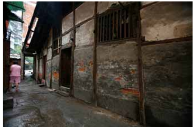
Figure 8 Brick-wood structure, Ms 8.0 Wenchuan Earthquake
