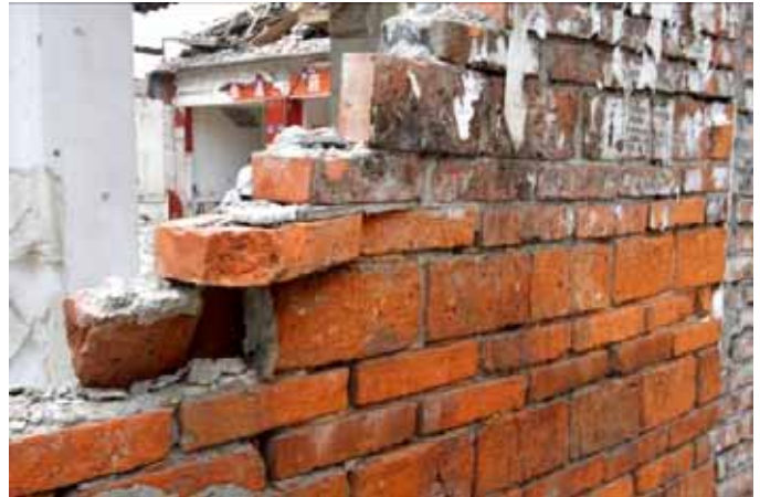
Figure 6 Brick structure, Ms 8.0 Wenchuan Earthquake
