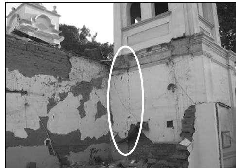
d) Vertical cracks on the intersection between the tower and walls
