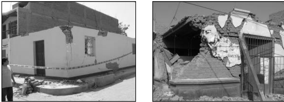
Figure 6 Diagonal and vertical cracks shown on corner buildings.
