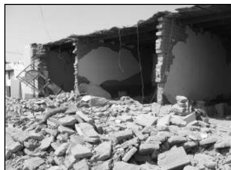
Figure 5 Collapse of the façade walls in adobe buildings.
