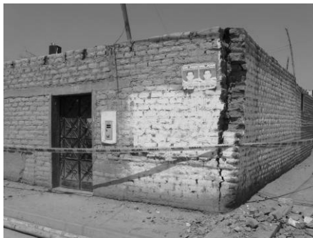
Vertical crack at corner of front wall
