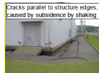
Figure 5. Cracks around incinerator building in TEPCO power plant
