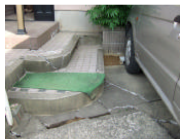
Figure 16. Damage to house
