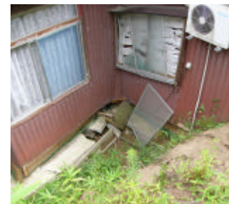
Figure 11. Lateral flow induced damage
