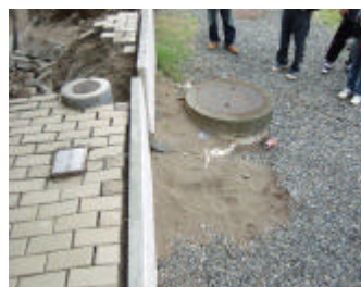
Figure 20. Uplifting of underground structures
