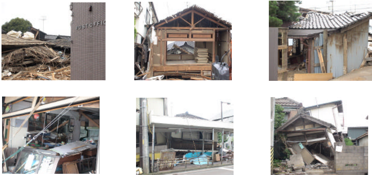
Figure 4. Damages to wooden residential and commercial buildings
