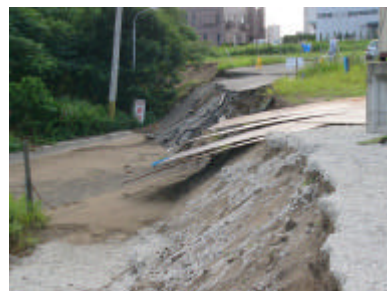
Figure 13. Lateral flow and subsidence
