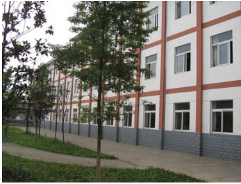
(Grade 0) No damage
