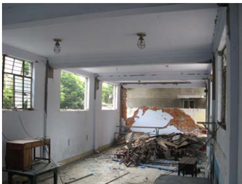
(Grade 4) Severe damage
