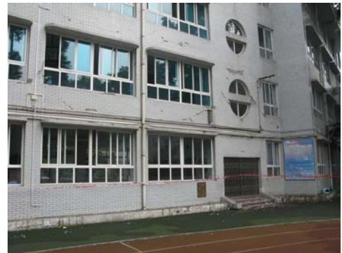
(Grade 3) Moderate damage
