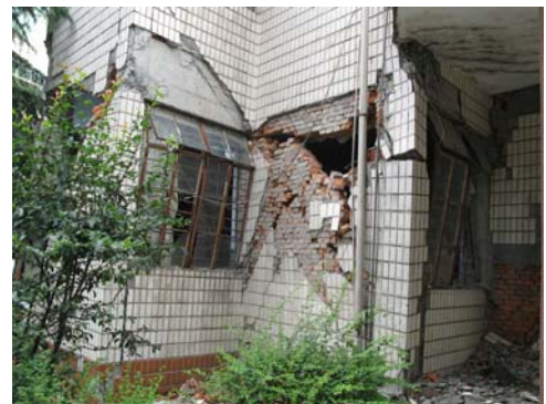
(Grade 5) Collapse or near collapse
