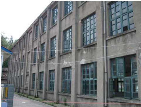
(Grade 2) Minor damage
