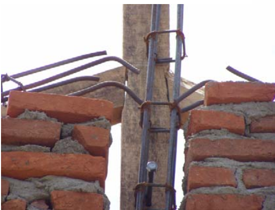
Figure14 Poor connection of rebar of RC framed
