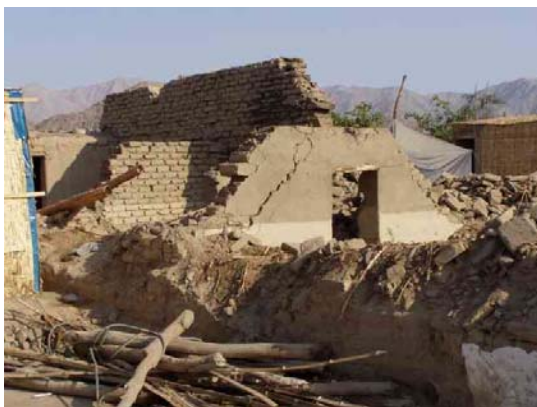
Figure6 San Jose de Los Molinos in Peru Almost all adobe houses were destroyed
