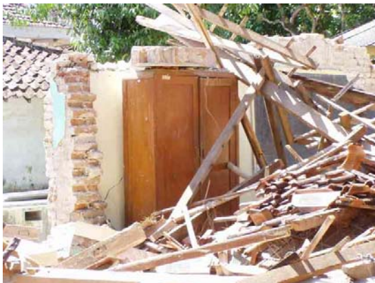
Figure1 Furniture remained standing even the building completely collapsed (Bantul in Indonesia)
