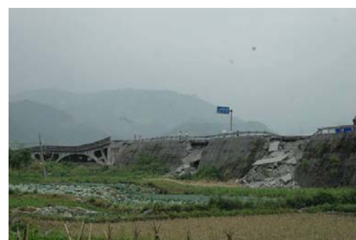
Fig.8 Fault rupture was observed
