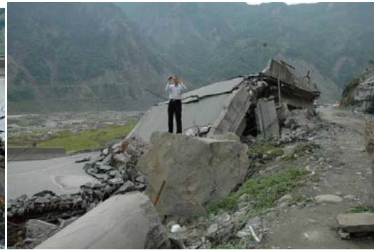
Fig.4 The falling slab of Baihwa Bridge
