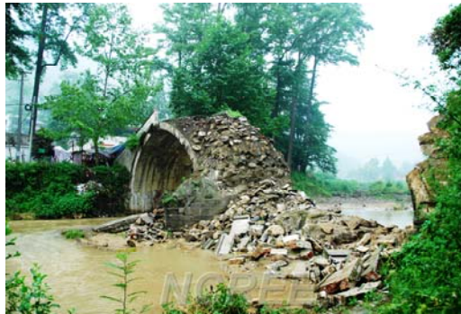
Fig.27 Collapsed arch of Bailu bridge
