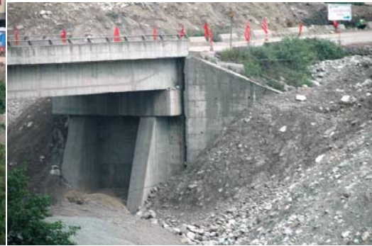
Fig.22 Damage on abutment
