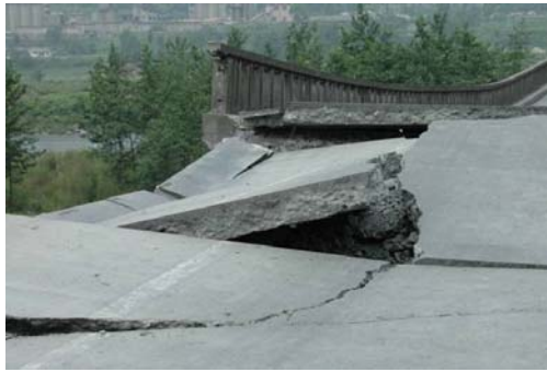
Fig. 9 Deck damage at approach
