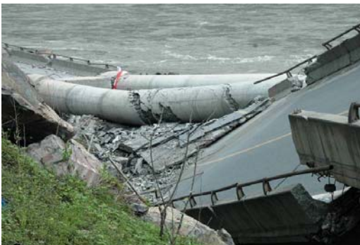
Fig. 5 The exploded pier of Baihwa Bridge
