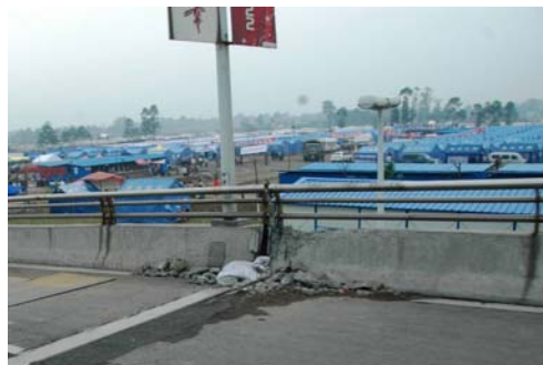
Fig.31 Expansion joint damage at Mianzhu
