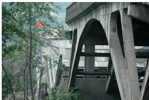
Fig. 13 The fallen spans of the Xiaoyudong Bridge
