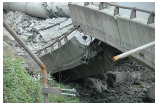
Fig.2 The broken slab and pier of Baihwa Bridge
