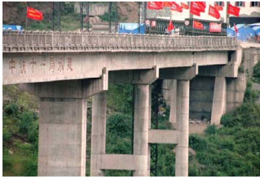
Fig.21 Damages on side stoppers
