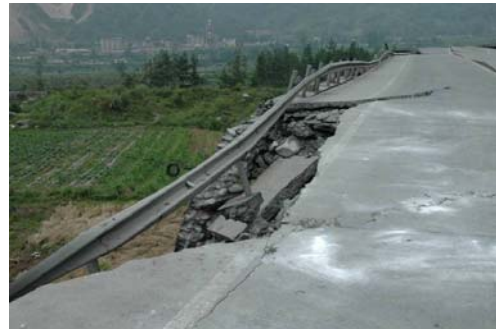
Fig. 10 Damage of the embankment
