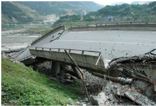
Fig.3 The falling slab of Baihwa Bridge
