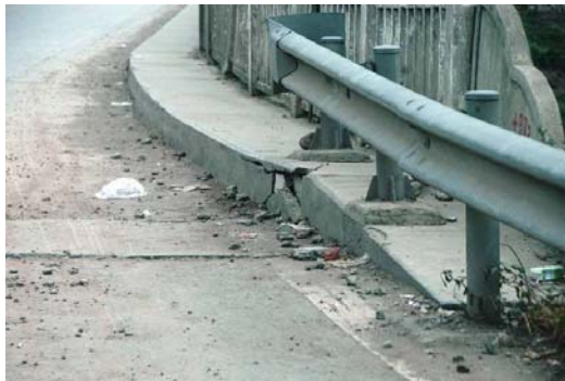
Fig.23 Damage on expansion joint
