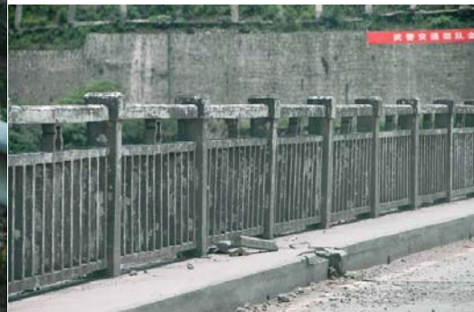
Fig.24 Damages on barrier and expansion joint
