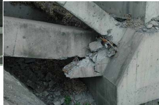
Fig. 12 Fracture at connection between arch and abutment
