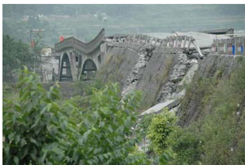
Fig.7 Damage of the Xiaoyudong bridge
