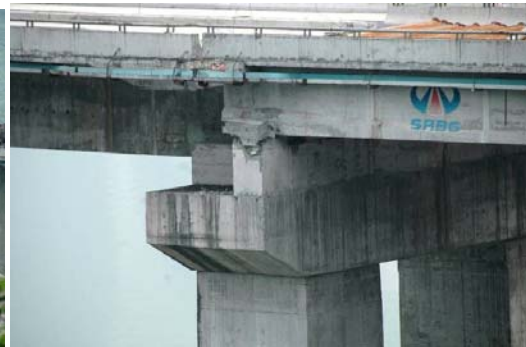
Fig.18 Damage of the side stopper
