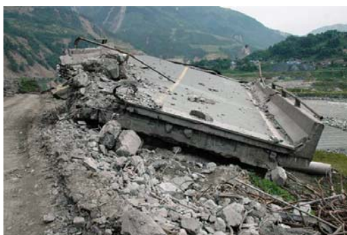
Fig.1 The falling slab of Baihwa Bridge
