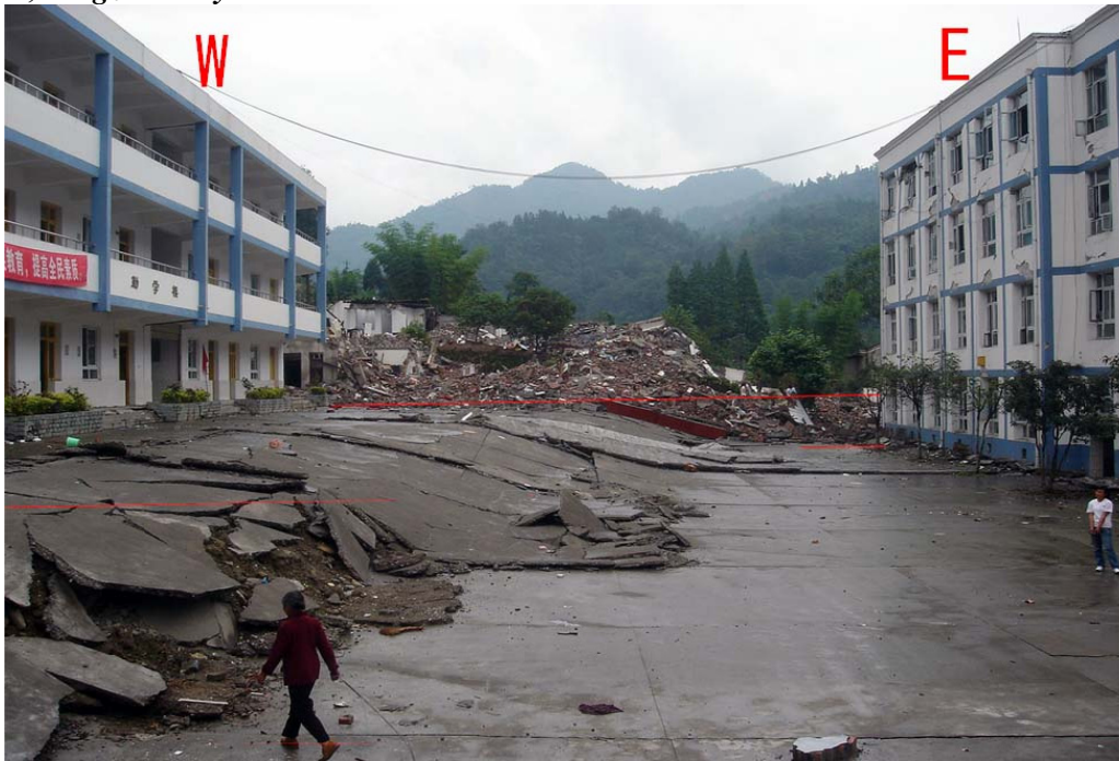
Figure 5 Looking north along the N00E-thrust fault with the maximum displacements over 2m in vertical, at Bailu zhen, Pengzhou City(Figure 1, Table 2.1). The new building W on hanging wall of the fault found no damages, while the old building E on foot wall of the fault suffered shear-stress cracks in X-shape.
