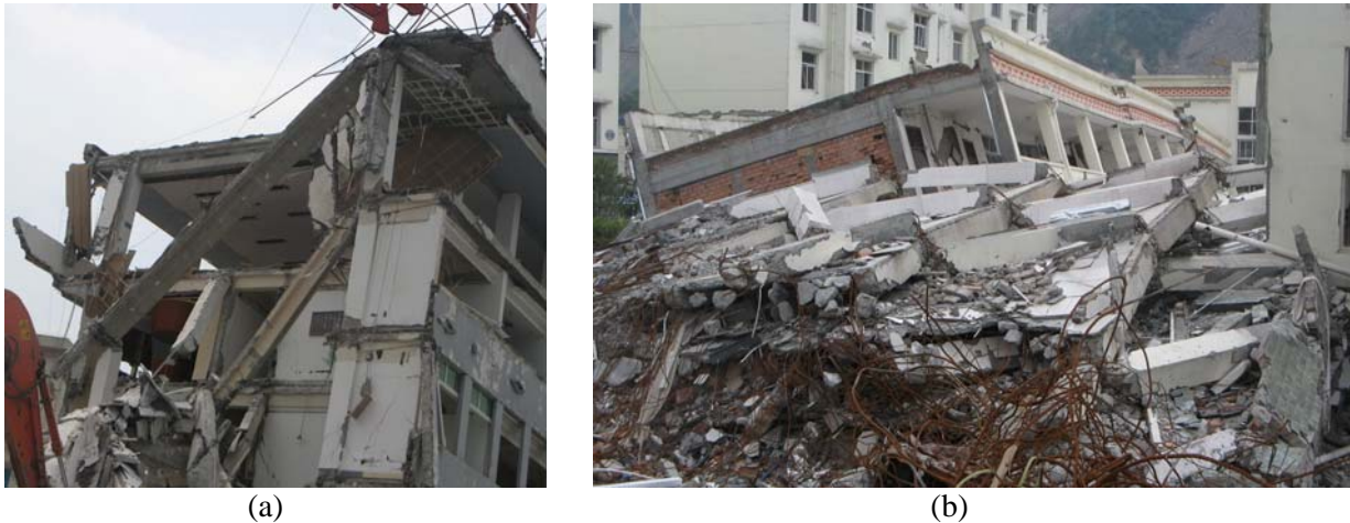
Figure 4 collapses of structures: (a) partially of an office building at Dujiangyan; (b) completely of one school building at Yingxiu (Adjacent building were heavily damaged)
